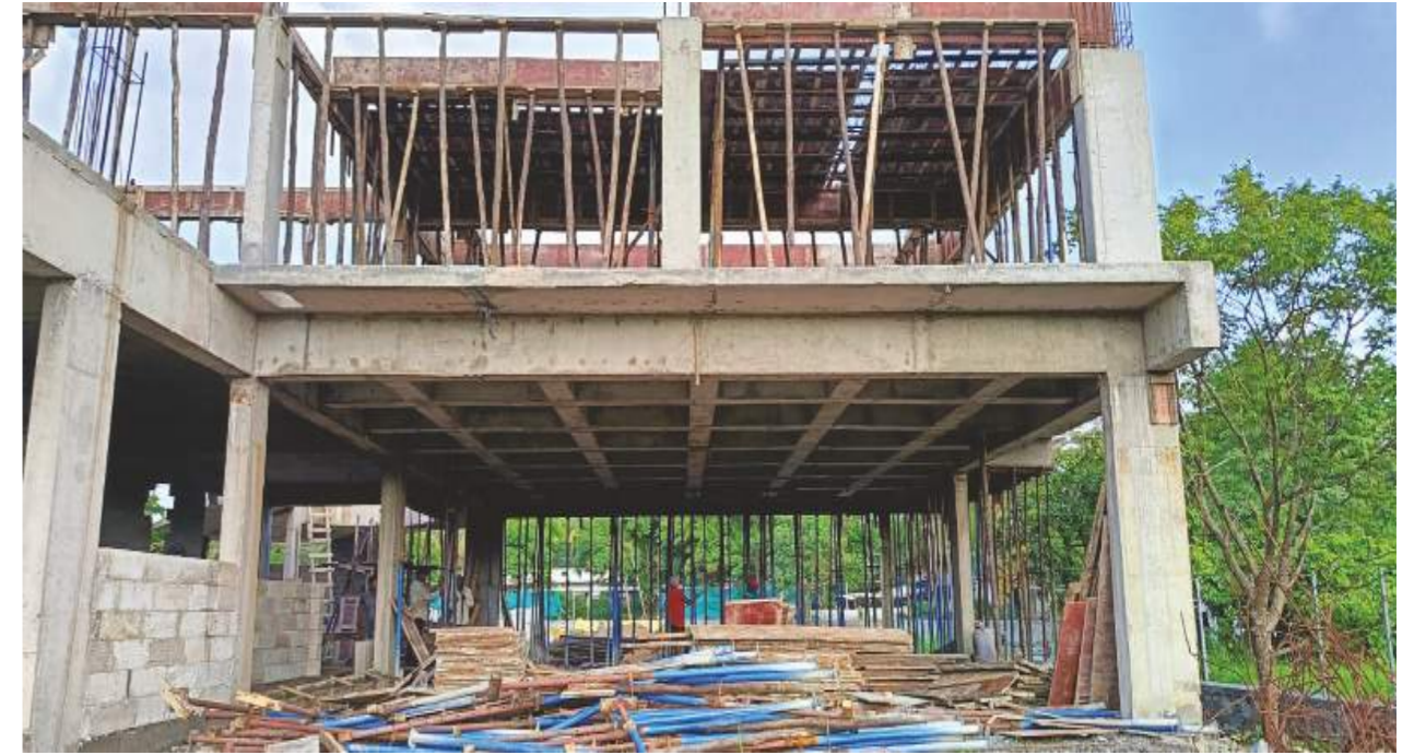
On site Development of first floor, also one can view grid slab construction.
